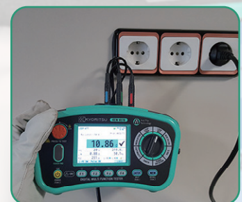
Loop test from a wall socket
